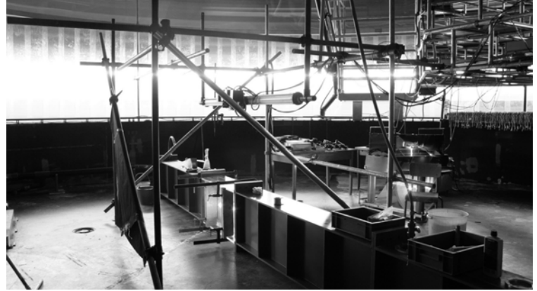
Figure 2: The duct mounted inside the turntable basin.
